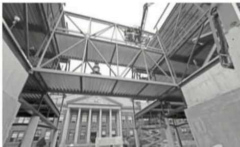
This construction is part of the expansion project at Port Chester High School. Port Chester passed a $79.9 million bond for a capital project. Their enrollment is up over 20% in the last decade and still growing. TANIA SAVAYAN/THE JOURNAL NEWS
